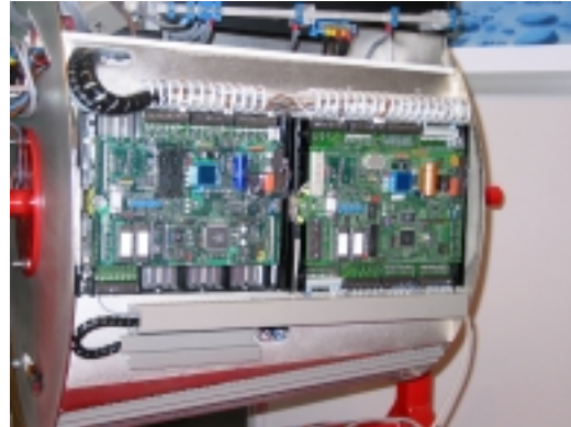
Fig.3.: Power Distribution Electronics
